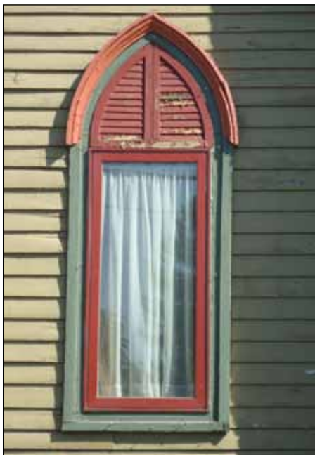
This window is the wrong shape, pane configuration and type.
