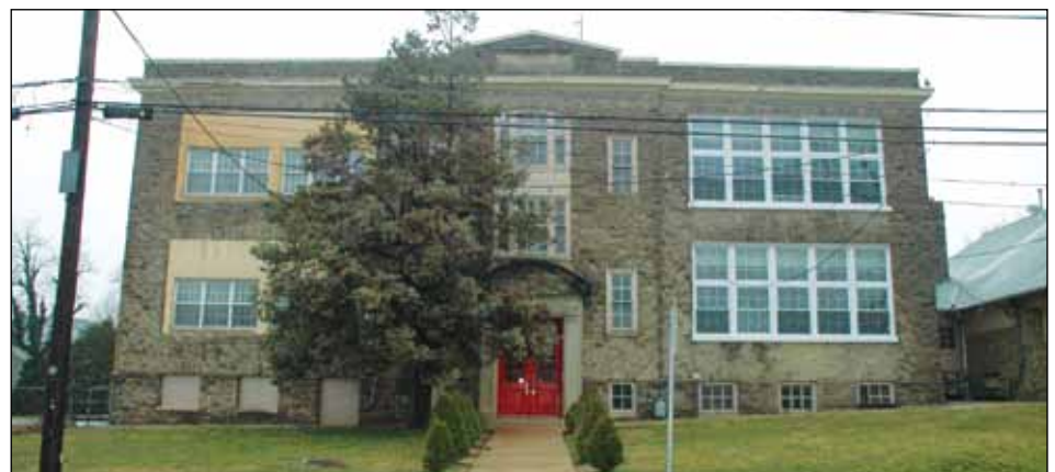
This historic school building is in its second cycle of window replacement. Those in the center bay and basement appear to be original. The windows on the left were replaced inappropriately with smaller windows that required alteration of the original window opening. The windows on the right, which are replacing earlier replacements, are restoring the size of the window opening and approximating the original pane configuration.
