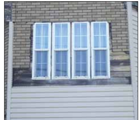
This window replacement used windows of the wrong size, shape and pane configuration for the window opening, and failed to maintain the existing trim.
