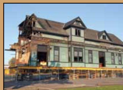
Partially demolished Depot on cribbing awaiting its new foundation. Cover photo of Pennsylvania At Risk in 2010.
