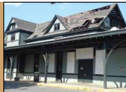
Dansbury Depot after the fire, before acquisition by the developer.
